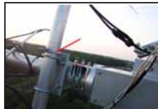
Here a vertical 10' mast with antennas weighing 30 lbs is inserted from above into a pair of muffler clamps and a single 2" UBolt (red line) prevents slippage allowing hands free work.
